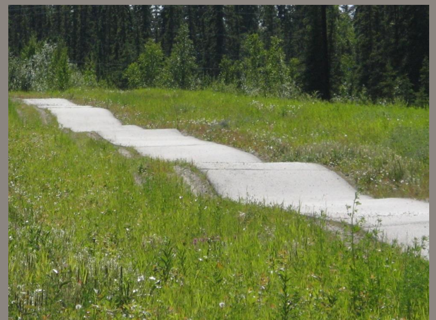
Bicycle path buckling due to permafrost thaw in Fairbanks, AK - Thomas A. Douglas, U.S. Army Cold Regions Research and Engineering Laboratory
