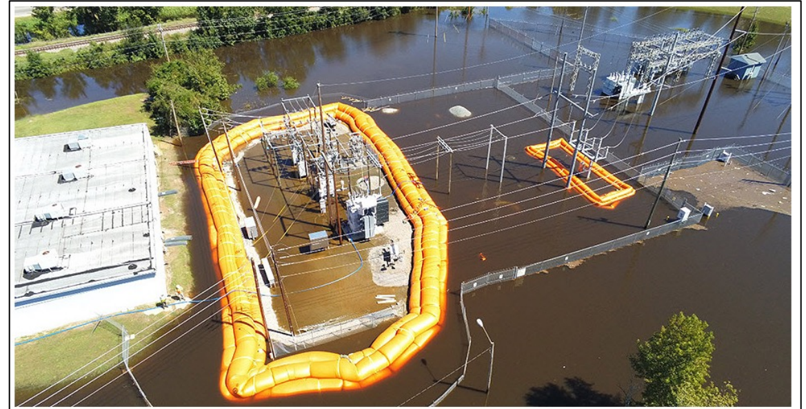
Portable flood-mitigation equipment surrounds a Duke Energy Corp. substation in North Carolina following Hurricane Florence. Duke Energy
