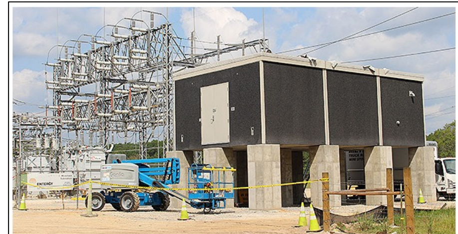
Entergy Corp. elevated a substation in Texas that was damaged during Hurricane Harvey. Entergy
