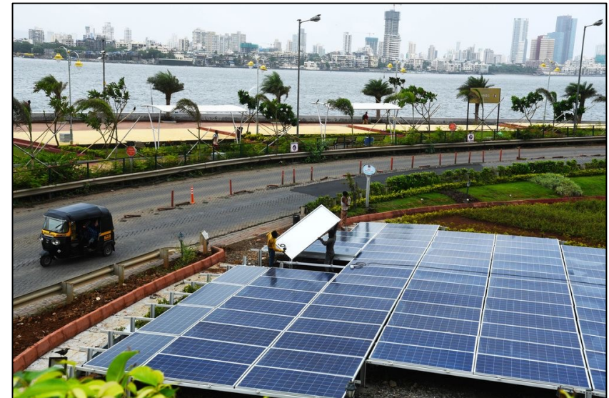
Solar panels installed in Mumbai, India. Source: Getty Images.
