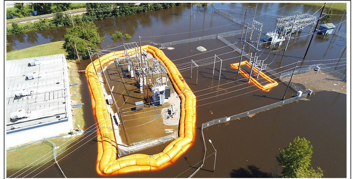
Portable flood-mitigation equipment surrounds a Duke Energy Corp. substation in North Carolina following Hurricane Florence. Duke Energy
