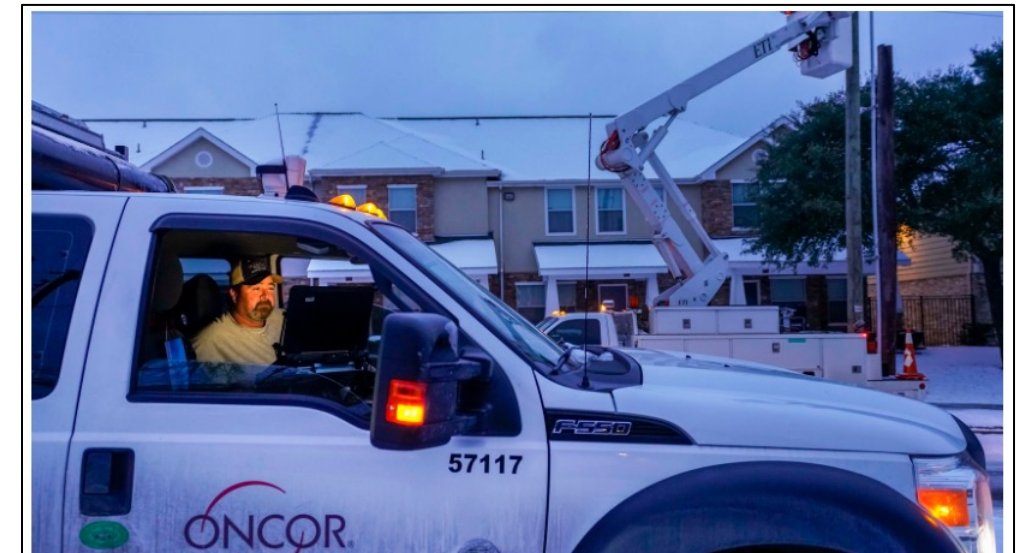
An Oncor crew works to restore power after the winter storm in Texas. Source: Smiley N. Pool/Staff Photographer/Dallas Morning News
