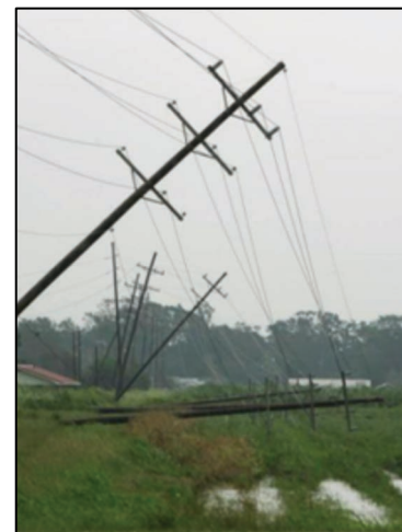
Powerline damage during Hurricane Gustav. Source: Matt Slocum/AP
