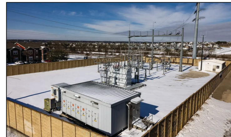
Texas power systems were unprepared for extreme winter temperatures. Source: Texas Tribune, February 2017
